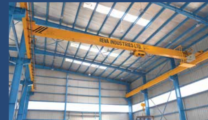
Reva Single Girder Cranes in Fabrication Shop
