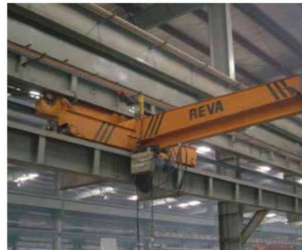
Wall Travelling Jib Crane 2T Capacity at Kirby Building
