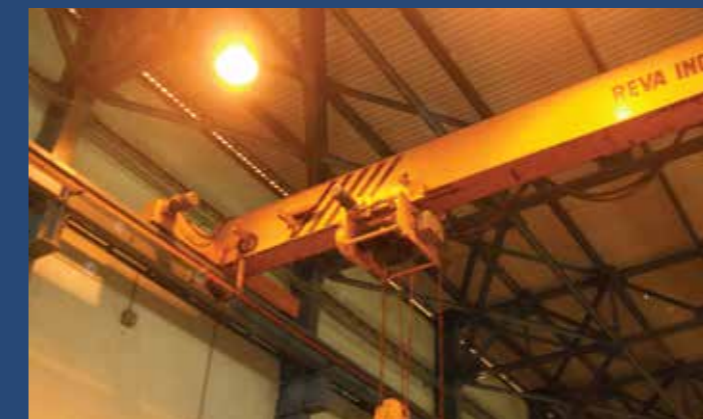
Reva Single Girder Cranes in Fabrication Shop
